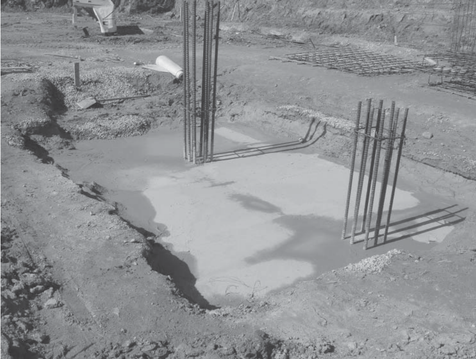
Combined footing (two column) after footing concrete is placed showing column reinforcing ready for splicing.
