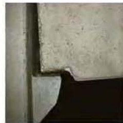
This concrete girder rests on the ledge that is assumed to act as a smooth contacting surface. (6)
