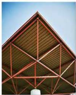
Typical roof-supporting space truss. Notice the use of ball-and-socket joints for the connections
