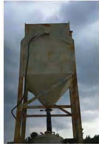
The walls of the tank must be designed to support the pressure loading of the liquid that is contained within it.
