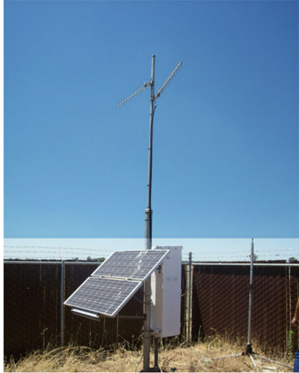
Fig. 6.3 GNSS CORS power supply and telemetry
