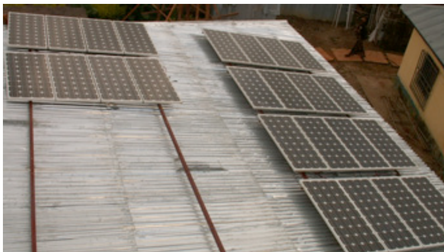
Figure 11.1: 24 solar panels with a nominal power of 80 W have been mounted to the roof of the NOC to provide power to the system 24/7.
