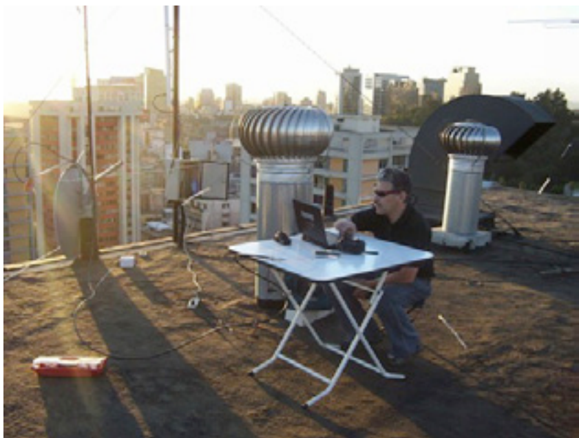
Figure 11.23: Downtown node connected to the Santiago southern node. Note the parabolic antenna for backhaul and the slotted antenna to connect the clients.
