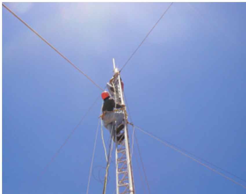
Figure 8.2: A climbable guyed tower.
