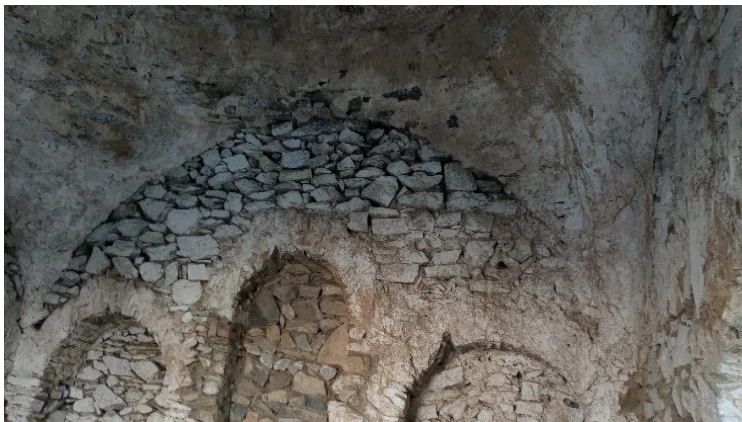
Interior pictures of the upper part of the Buddhist temple after renovation
