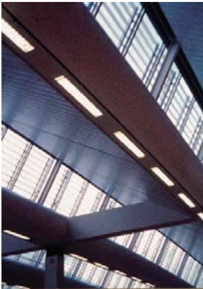
Detail of roof lighting
